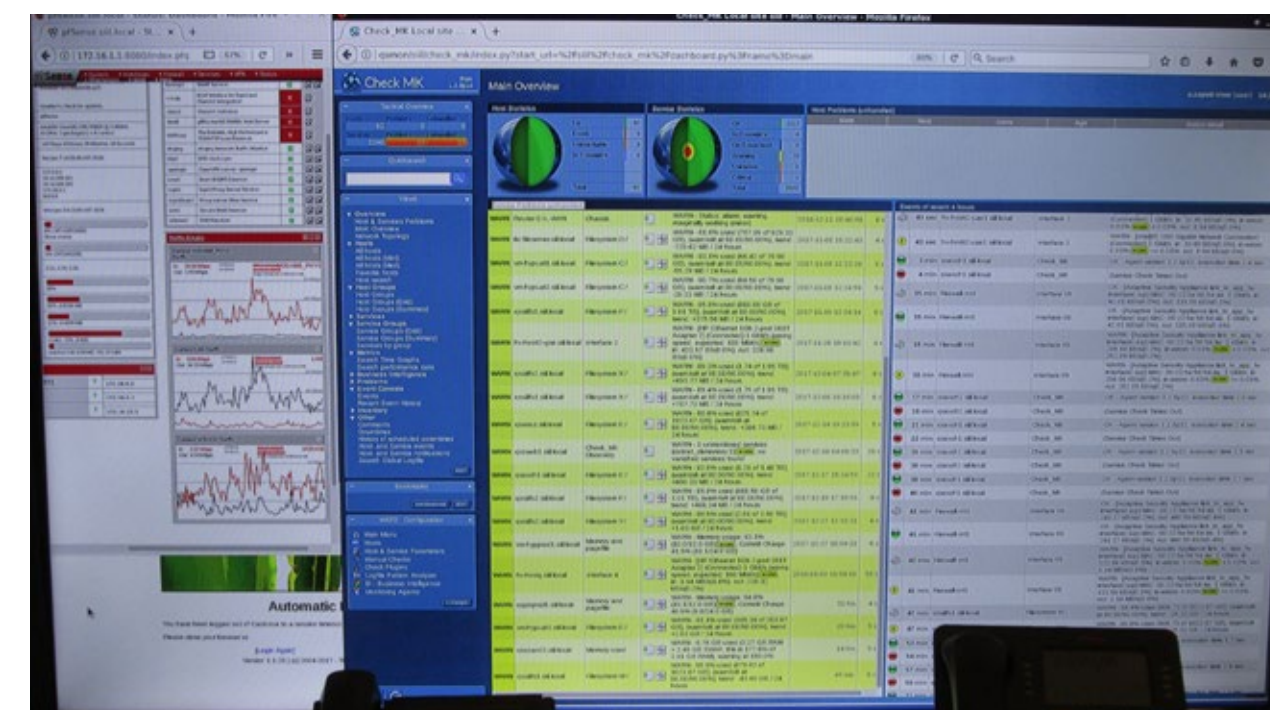
Real-time monitoring for SIIL servers, services, network and internet. Corporate IT are able to look out for potential problems and respond quickly to serious issues.
